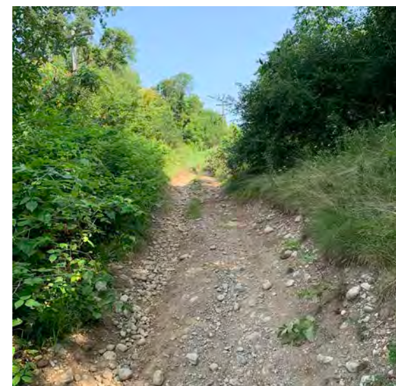
Image 23. A steep trail through an upland forest damaged from ATV use and erosion.
