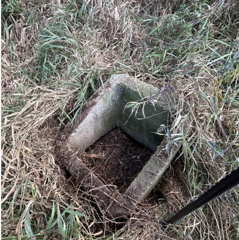
Figure 2 - Existing Concrete Catchbasin Filled with Sediment
