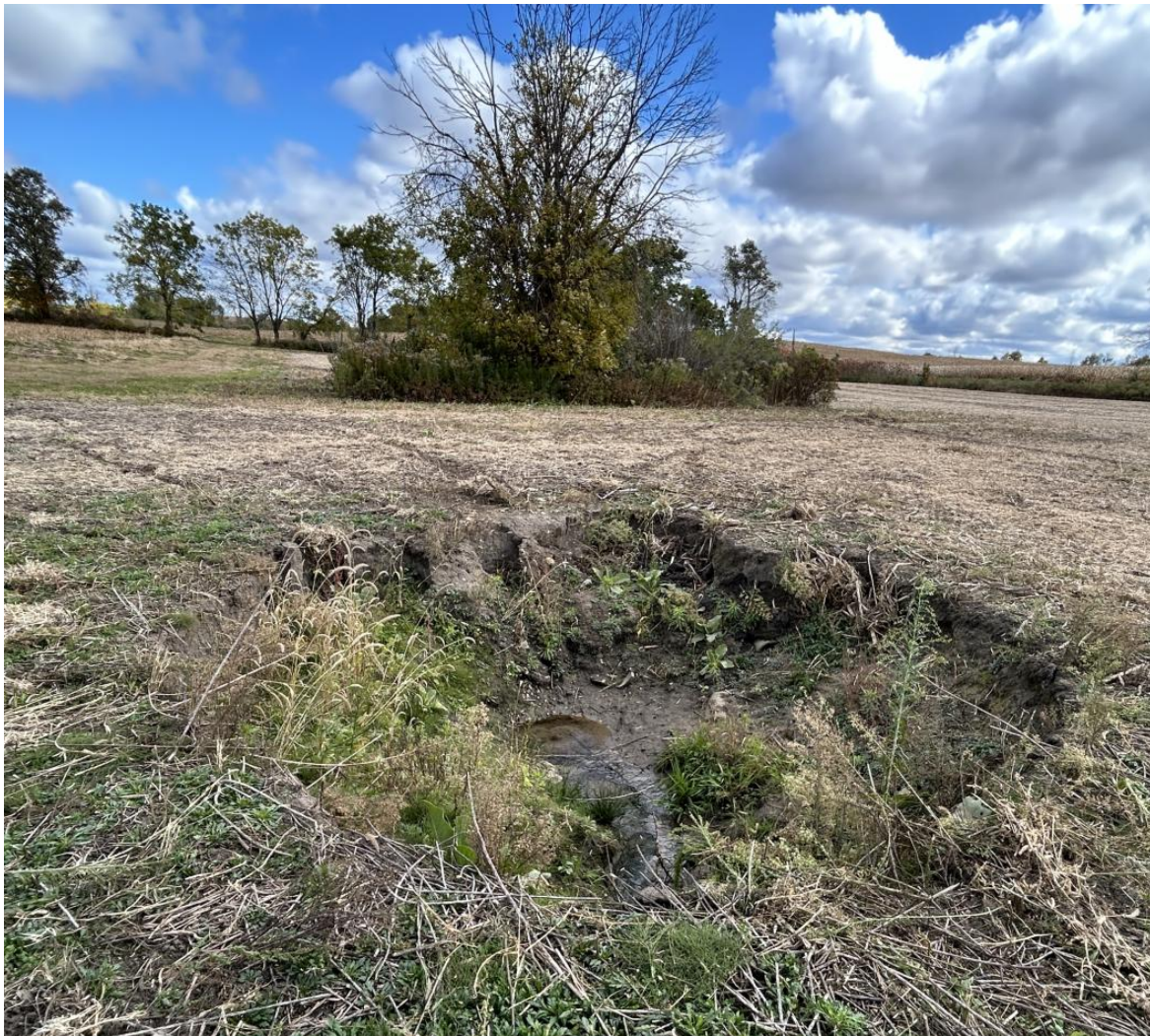
Figure 1 – Tile Blowout of the Terryberry Drain on Agricultural Lands on Lot 11, Concession 6
